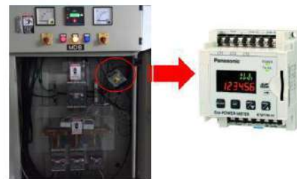
Fig. 4: The installation of Eco Power Meter to measure the amount of the electrical power used
